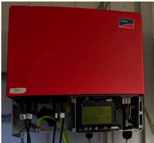
Figure 6: SMA SunnyBoy single phase inverter
