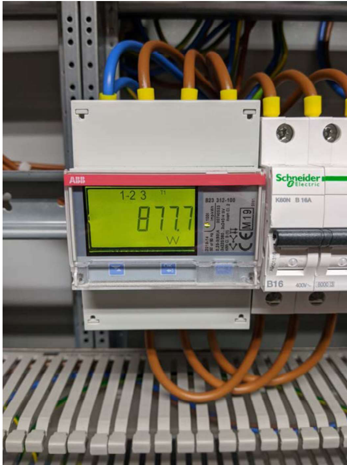
Figure 8: Bidirectional Smart Meter installed for each charging socket on CS#3
