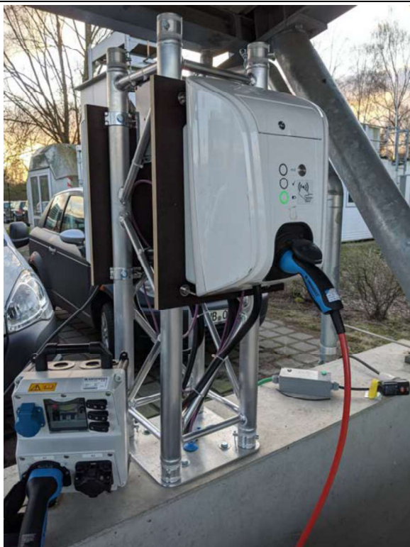
Figure 9: Wallbox prototypes installed on CS#3
