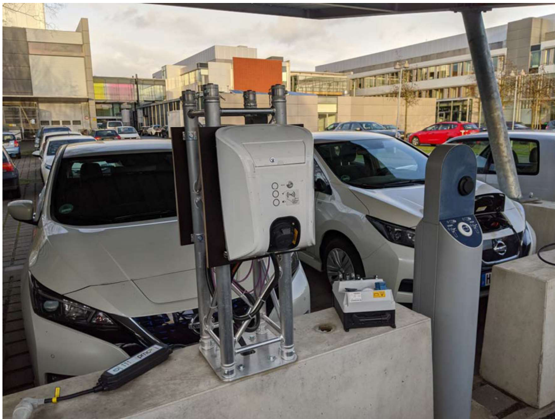
Figure 13: Prototypes installed on CS#3
