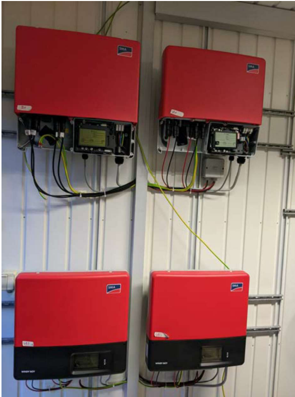
Figure 7: SMA WindyBoy (for batteries) and SunnyBoy (for PV) inverters feeding into 3 phase system
